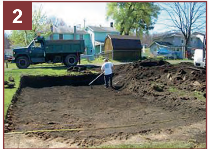
2 Additional digging so that site is level and gravel can be added.
